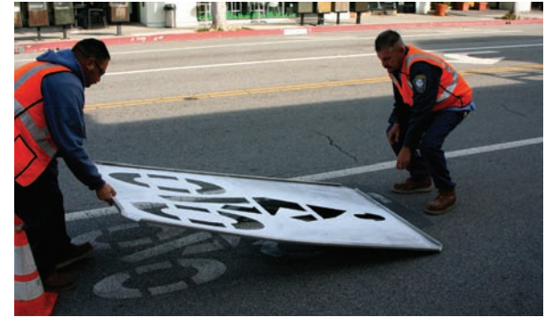
City crews install bicycle lane symbols and directional arrows. Source: City of Santa Monica
