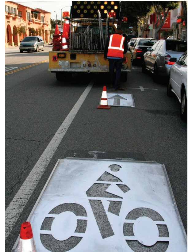
City crew installs bike symbols and arrows. Source: City of Santa Monica
